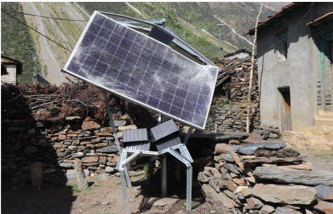
Figure 7: Shared solar home system in Darma Valley ( Damaged system)
