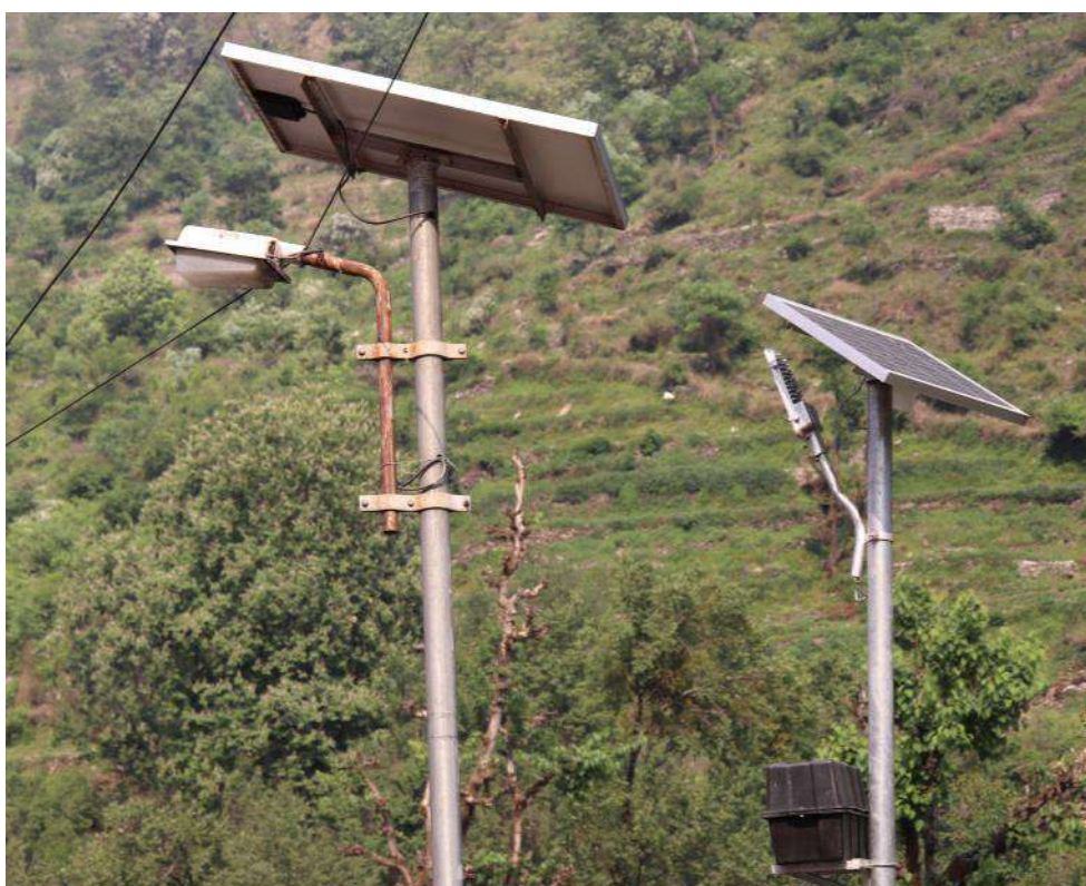
Figure 6: Solar street lights in Gangotri landscape (a defunct and a functional unit)
